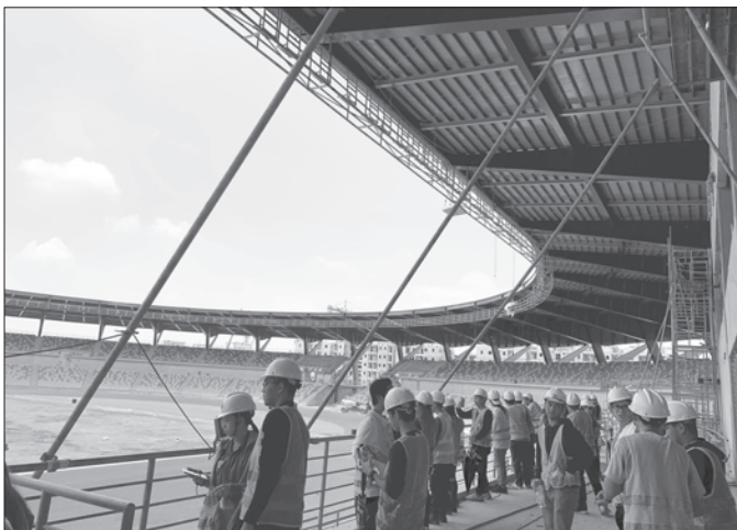
UC CE/Arch Seniors receive a full-fledged Briefing and a Tour of the Construction Site; courtesy of MTD Philippines CEO Engr. Isaac S. David.
